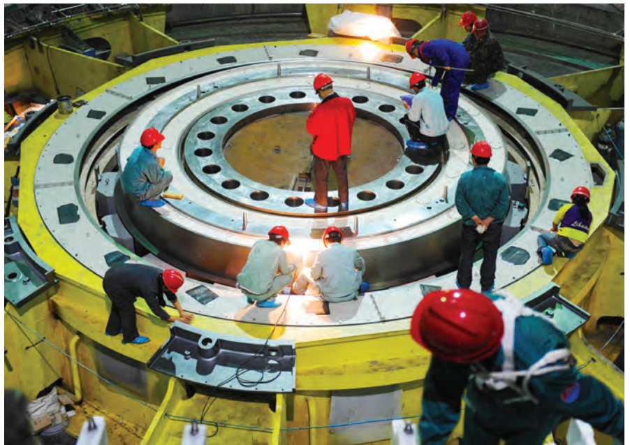
The rotor of the 1st generating unit of the Xiangjiaba Hydro-electric dam is made of 2100 tonnes of martensitic stainless steel Copyright © Sina Corporation, All rights reserved
