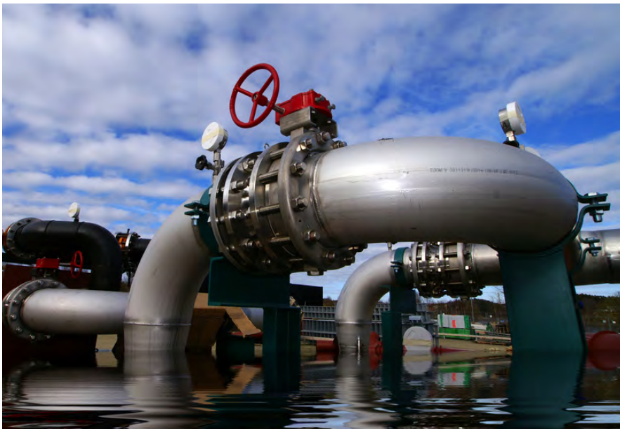
Industrial zone, stainless steel pipelines and valves
